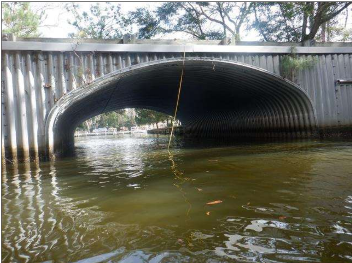
Span 1 Culvert Section 1: PRIORITY ACTION REQUESTED - 2' VERTICAL EXPOSURE OF TOEWALL ON WEST END
