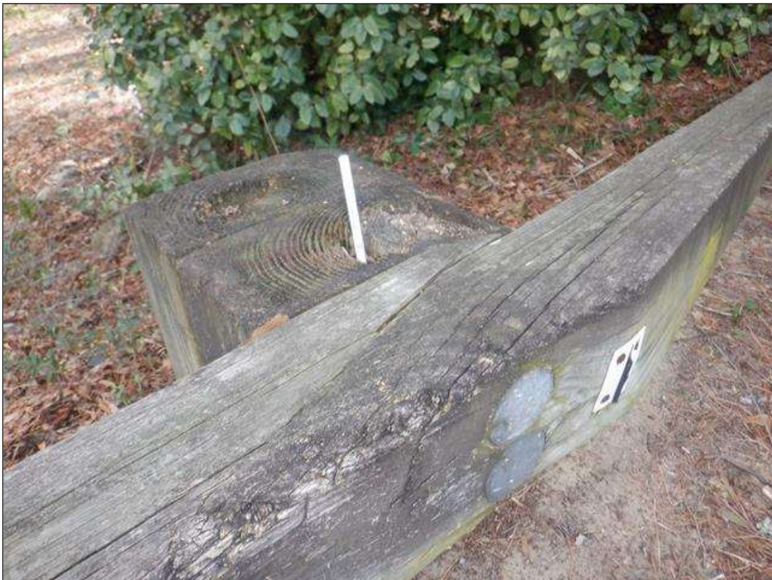
RAILING POSTS HAVE END DECAY TO 1" DEEP.
