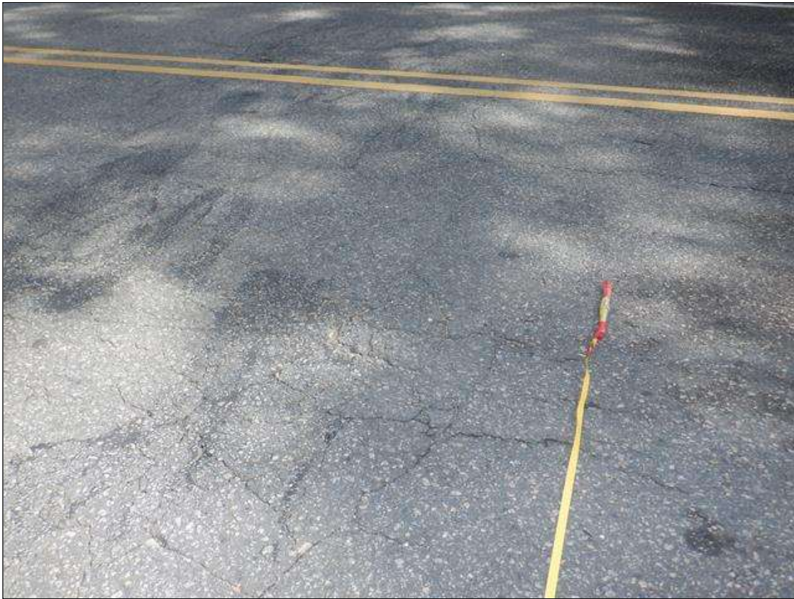
AWS - CRACKED TO 1/8" AND SETTLED TO 1"
