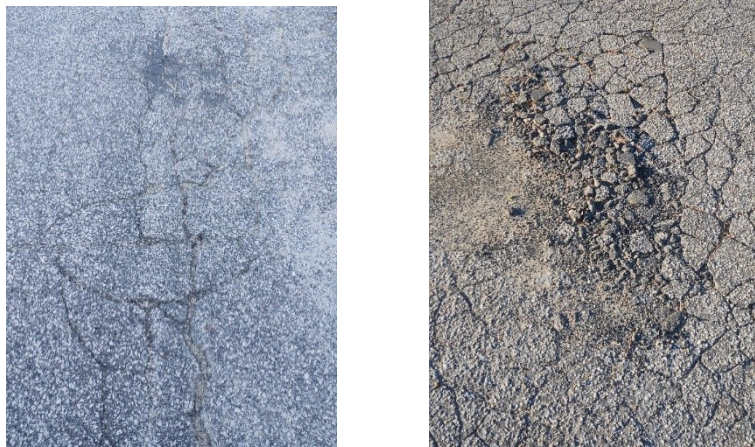
Figures 3 & 4: Fatigue Cracking as seen on First Avenue and Mizzen Mast
