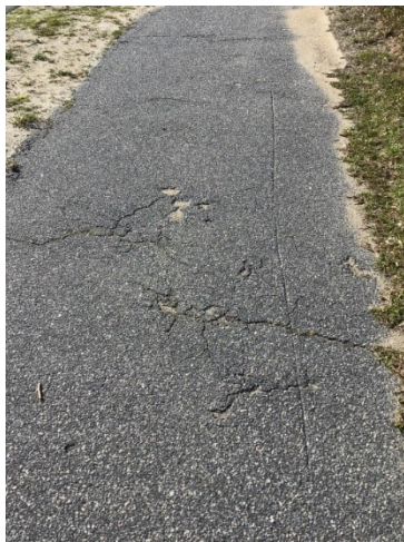
Figure A - Transverse Cracking
