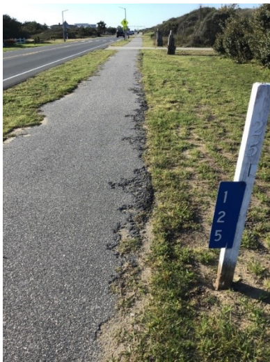
Figure E – Raveling of asphalt edges
