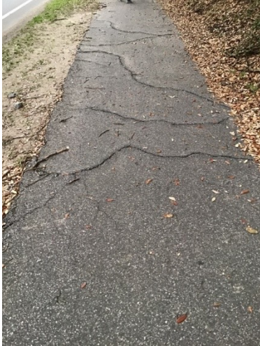
Figure C – Root intrusion cracks
