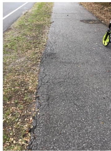
Figure B – Edge Cracking
