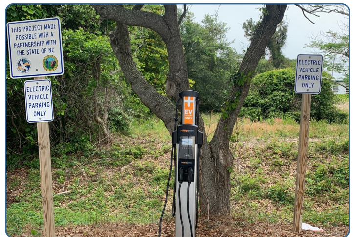
Electric vehicle charging stations located at Town Hall.
