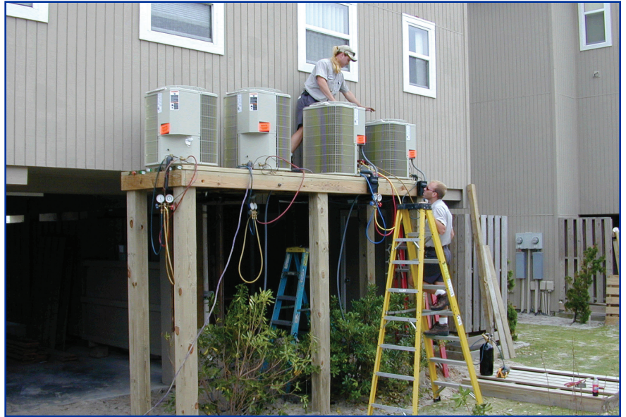
Elevated air conditioning compressors.
