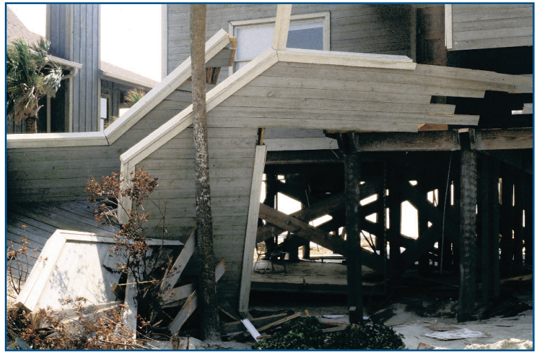
The rails on these stairs were enclosed with siding, presenting a greater obstacle to the flow of flood water and contributing to the flood damage shown here.
