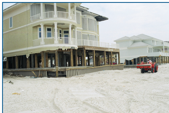
Breakaway walls that failed under the flood forces of Hurricane Ivan.
