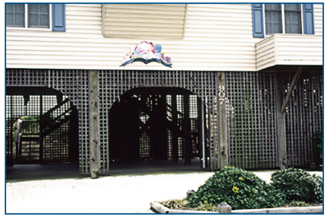
Open wood lattice installed beneath an elevated house in a V zone.
