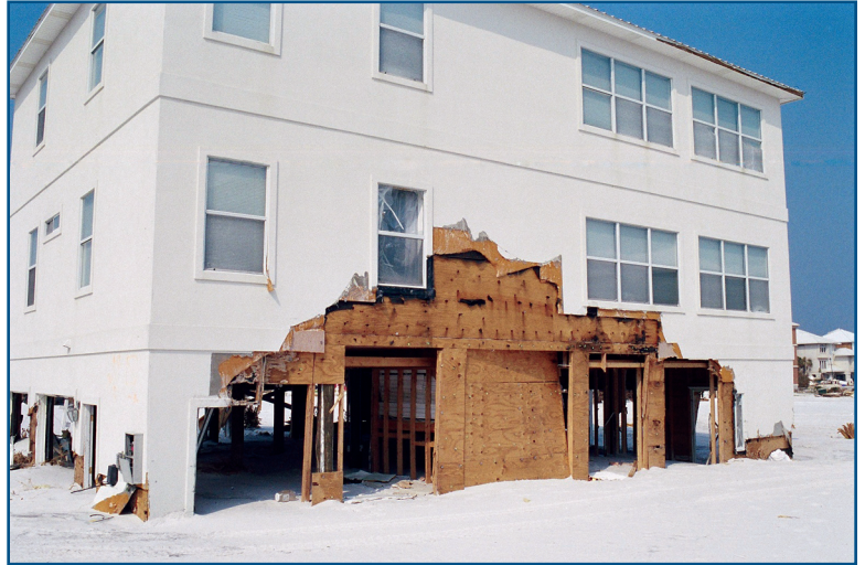
Siding on the non-breakaway portions of this elevated building was extended over breakaway enclosure walls and was damaged when breakaway walls failed under flood forces.
