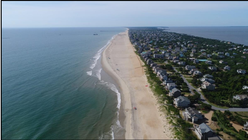
Figure 7. View of the completed Town of Duck project, looking south from north of the project.
