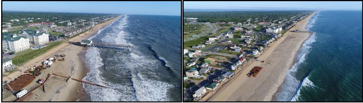
Figure 10. View of the beach nourishment project within the Towns of Kitty Hawk and Southern Shores, looking north - Pre-Construction (left), Post-Construction (right).
