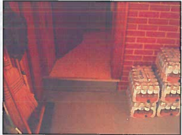
The Apparatus Bay Restroom is not accessible due to a step up, knob handle, and the accessible route clearances are encroached upon by equipment and water bottles.
